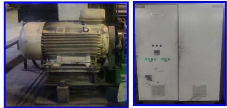
Energy Efficient IE-3 Motor with VFD Panel
